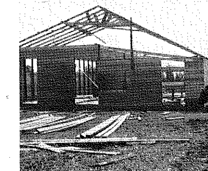
In carrying out its community service project, one F.F.A. chapter constructed a chicken house for a needy family
