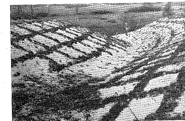
The sides are sloped and sod stripped to permit vegetation to become established. —Photo by U. S. Soil Conservation Service.
