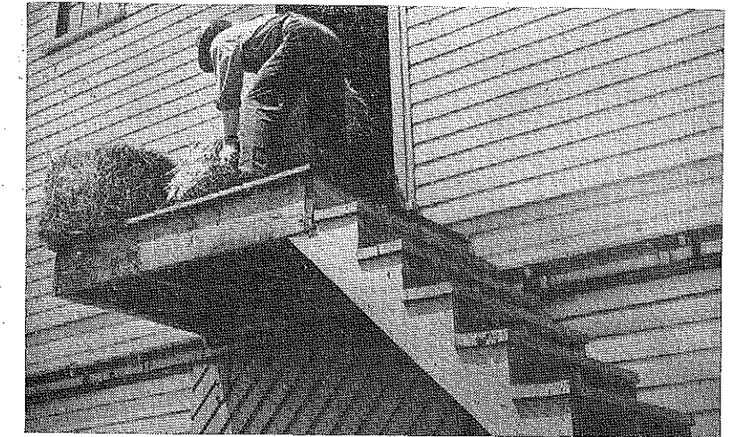
No guard rail on stairway to barn walk, a common hazard which contributes to falls, the leading cause of farm and home accidents.
