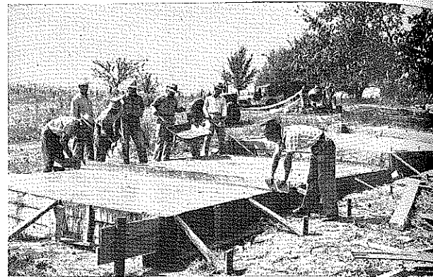
Group of on-farm training class at Marshall, Missouri, obtaining participating experiences in laying foundation for granary. Pictures of this sort are useful to the local press and to outside publications.
