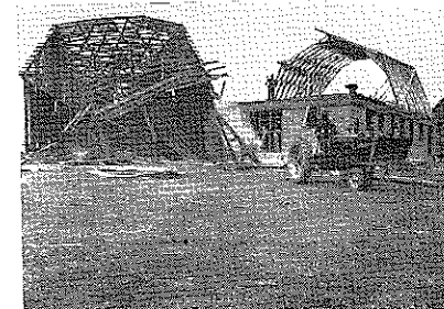
An old tobacco barn was torn down and help was given in the construction of a dairy barn during the work-day on the Higgins farm.
