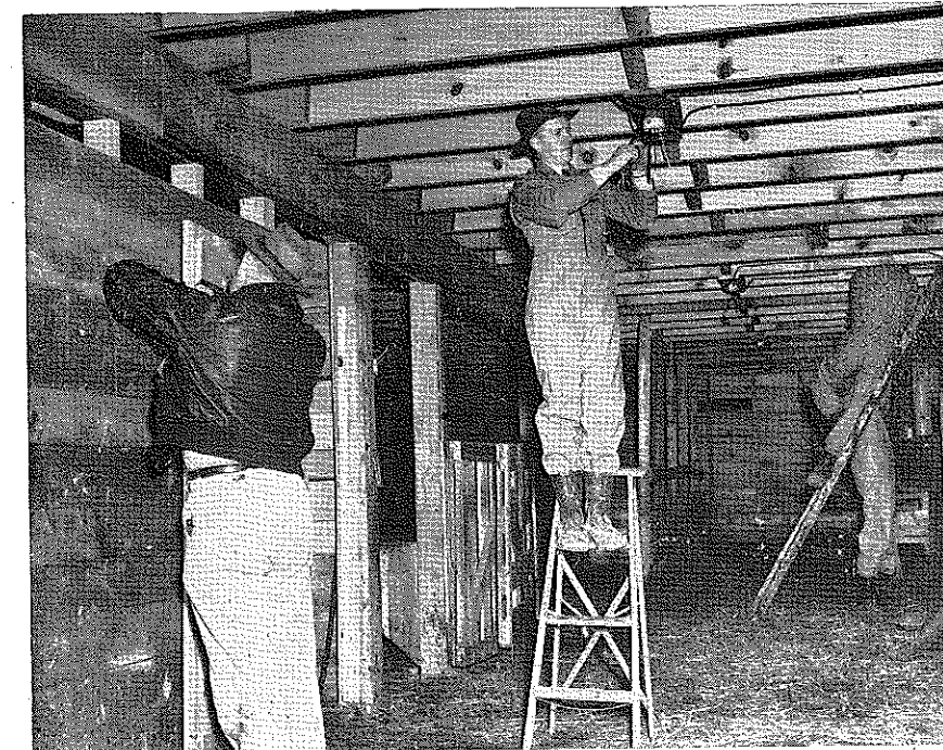
Carrying the instruction through the doing phase here are the teachers at work installing the wiring system in a barn after it has been completely planned and approved for installation. Service entrance and six circuits were installed.
