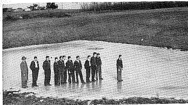
A farm pond constructed by a Vo-Ag class. The local S.C.S. technician assisted in planning the pond.
