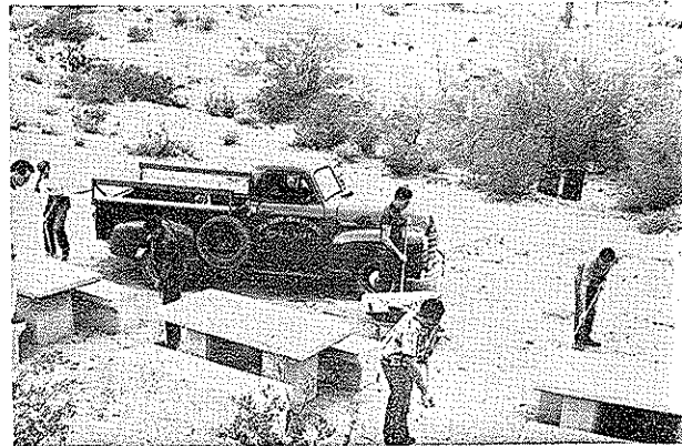
→ This community picnic site is being constructed as a community service project by an FFA Chapter in Arizona. Another example of combining opportunity for desirable learning with community improvement.
