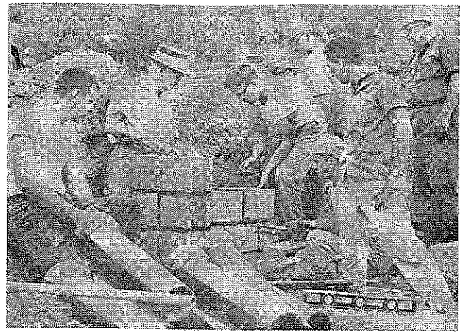
Photo A—Pennsylvania teachers of vocational agriculture begin work on a 24 ft. x 40 ft. garage and machine shed as part of an in-service teacher education workshop.
