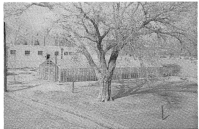
This 20 X 80 feet plastic covered greenhouse was constructed by students in less than 10 days. Scrap boiler pipe, obtained from the school system, was used in the basic frame, along with new lumber. The entire greenhouse was built at a cost of less than $1500.00.
