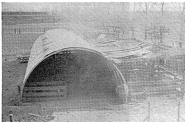
Students poured the foundation for this surplus 20 X 56 foot quonset-type building purchased for $250.00. The completed building is used for the farm flock of Rambouillet sheep.
