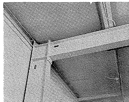
Roof structure design, insulation and smooth interior wall surface are shown in this picture.
