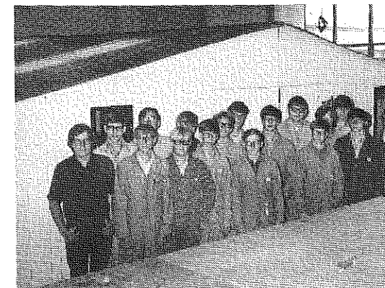
A pull-together hog house is a building project that we can make in two sections and move out through our 12' x 16' door. This was constructed for one of the boys in our class. In the foreground is a large sectioned platform for the Nobles County Fair Board.
