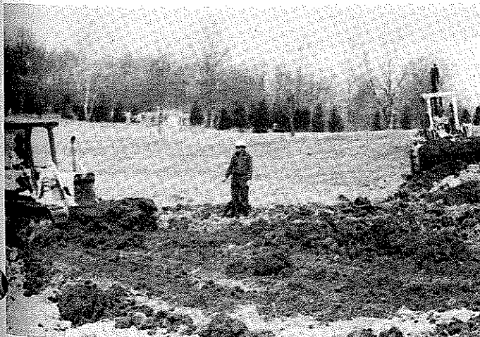
Conservation students are constructing a pond under the supervision of Conservation Instructor — Donald G. Farrand.
