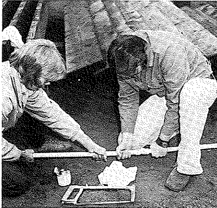
Two students at Operation Green Thumb assemble plastic pipe for a sprinkler irrigation system.
