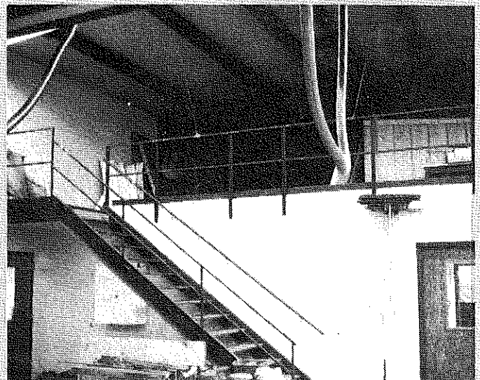
Many departments have effective storage by utilizing overhead spaces. Permanent stairs, railings and kickboards are essential for safety in such areas. Care must be taken to provide appropriate lighting and to manage such areas carefully to avoid hazards to students.
