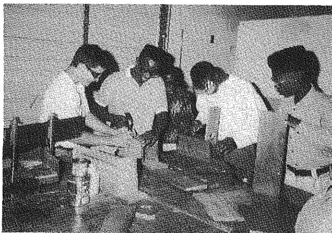
Simple hand tools are used to build houses at the completion of a unit on Natural Resources. Such activities teach self-confidence and pride in workmanship.
