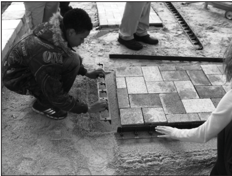
Gettysburg Area High School students installing edging materials to hold pavers in place. Read the complete article starting on page 19.
